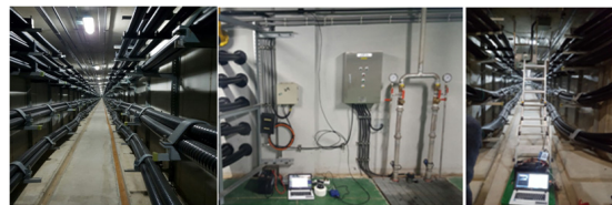
Fig. 7 Actual internal and demonstration test of underground utility tunnel
