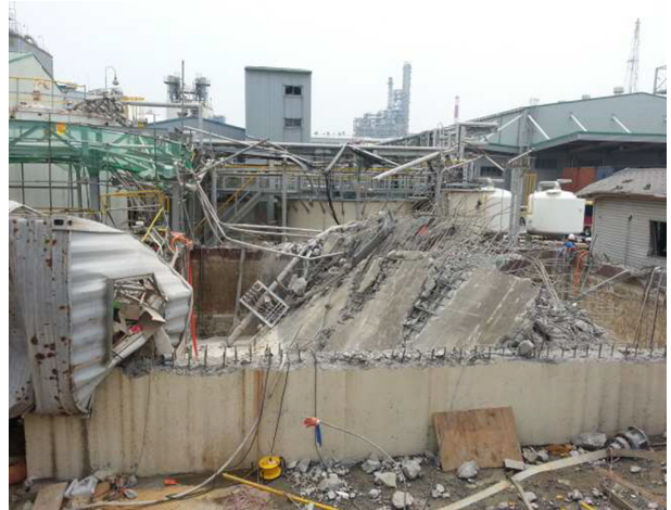
Fig. 3. Picture after explosion of waste water pond.
