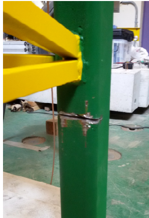
Fig. 9. Inflicted damage (Case 2)
