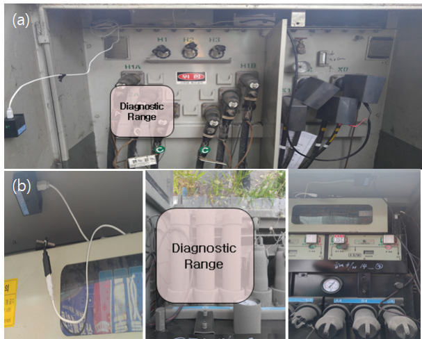
Fig. 10. Photograph of field installation.
