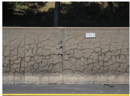
(a) Deteriorated concrete median barrier
