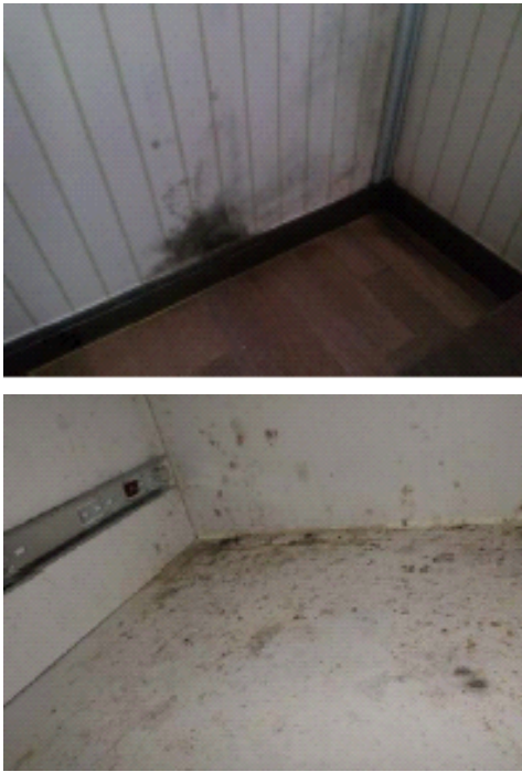
Fig 1. Examples of condensation in walk-in closet
