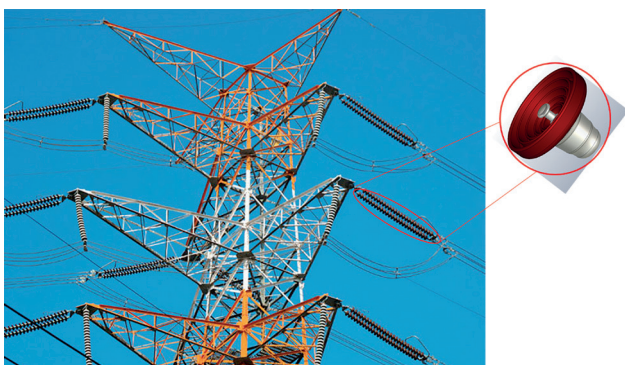
Fig. 2. Suspension-type porcelain insulator used for 154 kV and 345 kV power transmission lines in South Korea.
