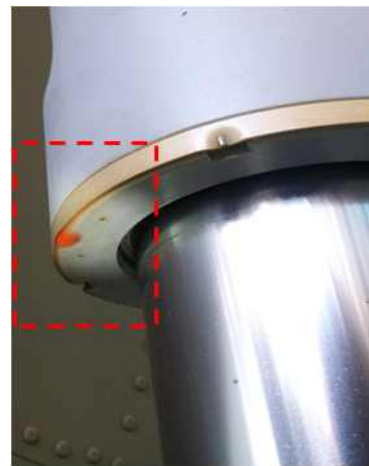
Fig. 7. External hydraulic fluid leakage
