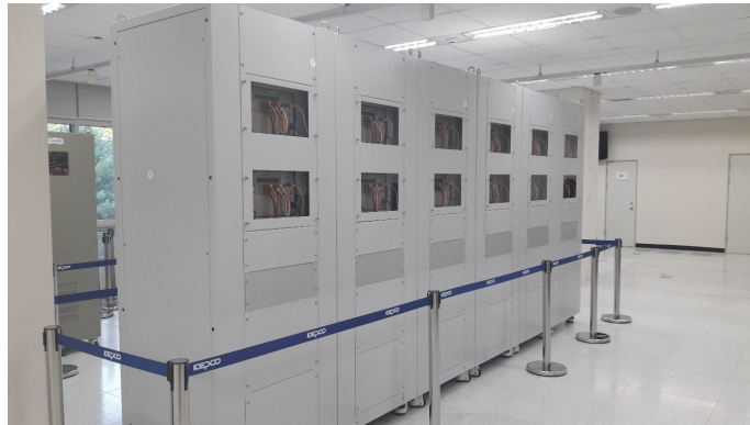
Fig. 4. Interface amplifier cubicles.
