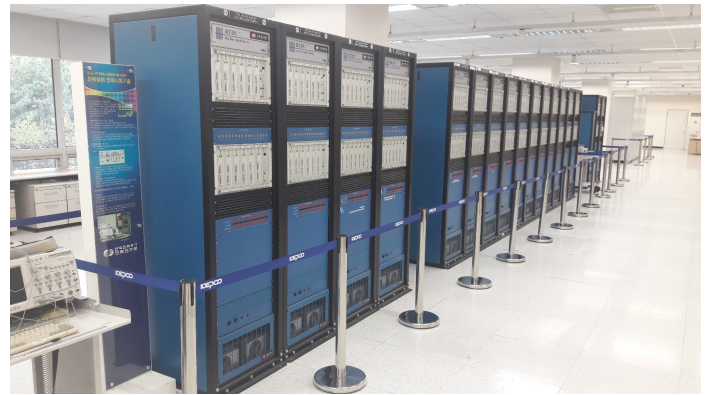
Fig. 5. Upgraded RTDS in KEPS lab.
