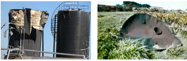
Figure 14. Damaged asphalt storage tank and roof of tank flying because of blast pressure.
