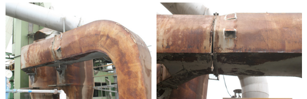
Figure 6. Damaged and expanded first smoke duct.
