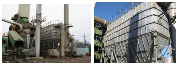
Figure 9. Expanded bag house filter.
