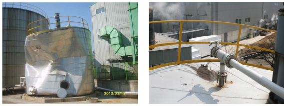
Figure 12. Damaged and overflowed asphalt tank.
