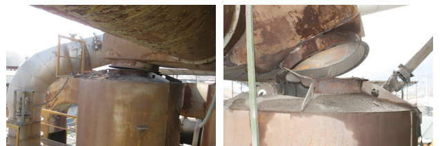
Figure 8. Cyclone that connection part was bolted with secondary smoke duct.
