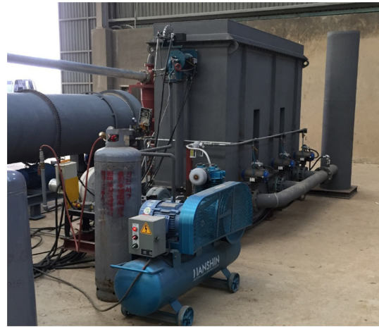
Fig. 4. Regenerative thermal oxidizer (RTO) for decomposing the volatile organic carbons emitted during drying process.
