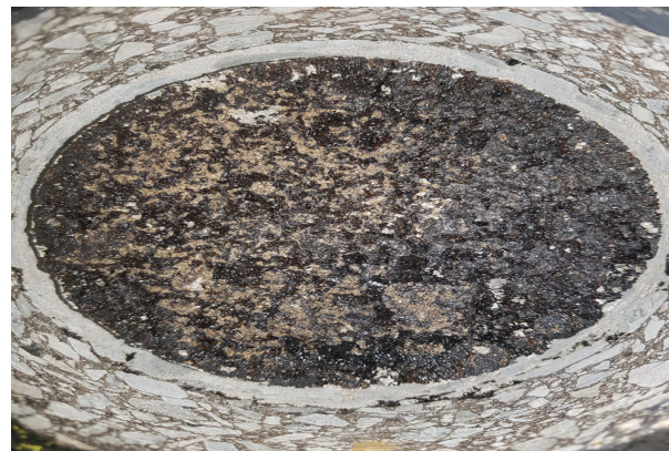
Fig. 8 Bonding Failure Surface (Bottom of Core)
