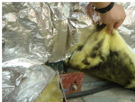
Fig. 1 Condensation problems around the fastener of curtainwall system.
