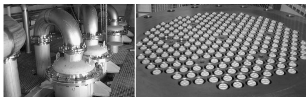
Fig. 5. Industrial pilot plant for dewatering of ethanol with NaA-membranes of Fraunhofer IKTS. Reproduced from[15] by permission of John Wiley and Sons Inc.
