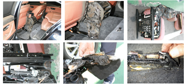
Figure 6. Case that a fire broke out because a DGL got between driver sea trail.
