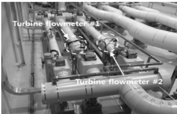
Fig. 8 Photograph of turbine flowmeter for flow test
