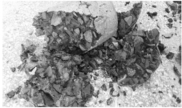
Fig. 14. Expansion failure of ACC-50
