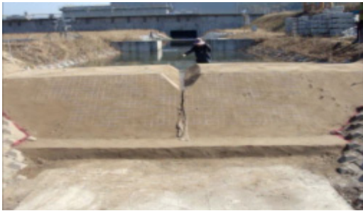
(a) Local scour occur due to overflow
