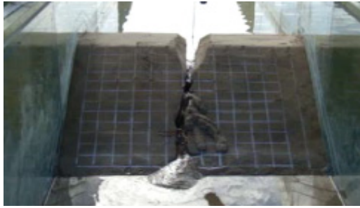
(a) Local scour occur due to overflow
