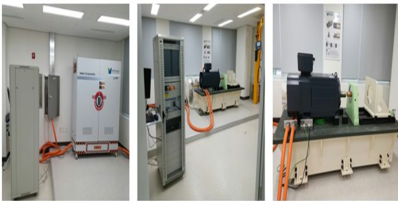
Fig. 7. Installed Marine environment simulator.
