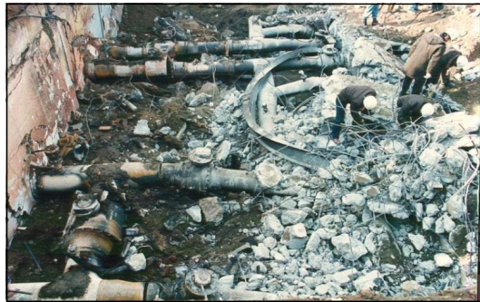
Fig. 2. Accident of city gas governor
