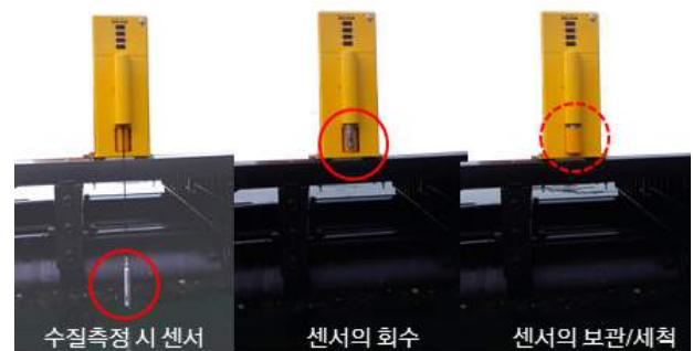
Picture 5 Operation method of non-cleaning measuring equipment using a pulley
