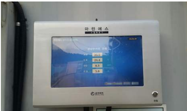
Picture 7 Installed display
