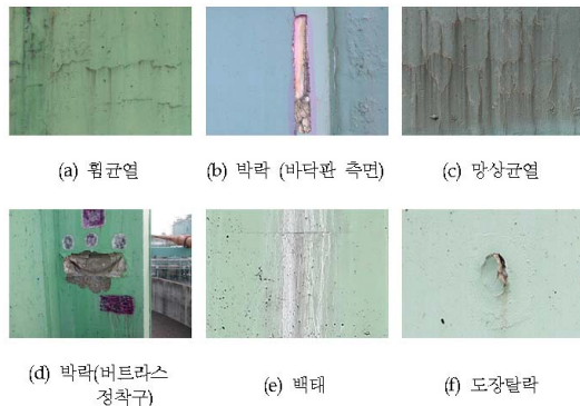
Fig. 4. Kinds of damages for the wall of LNG storage tank.
