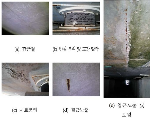
Fig. 5. Kinds of damages for slab and support equipment of LNG storage tank.
