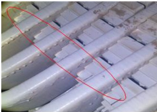
Fig. 2. Efflorescence near the winding slot withdrawal part.
