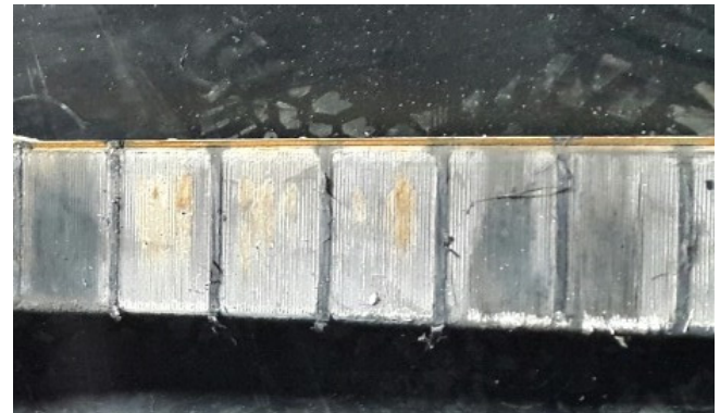
Fig. 4. Abrasion condition of the surface of stator windings.
