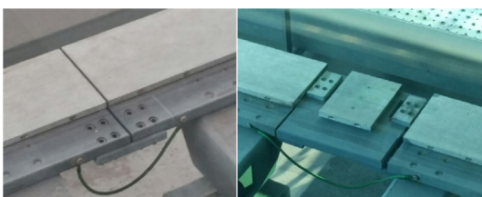
Fig. 1 Pictures of guideway joints. Some of them are joined by intervening plate as shown in the right picture
