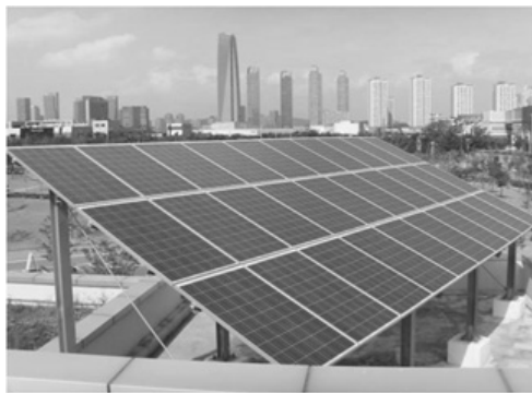
Fig. 1 6 kW grid-connected photovoltaic system
