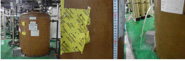
Fig. 6. Real pictures for a leakage experiment to verify the results of simulations.
