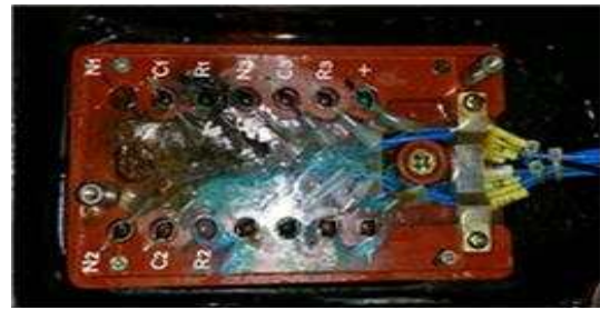
b) corrosion of connection
