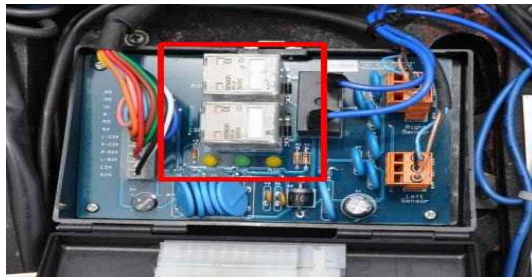
a) failure of control part
