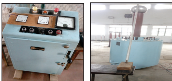
Fig. 2. Primary and secondary sides of transformer in lab to apply high voltages to the electrode system.
