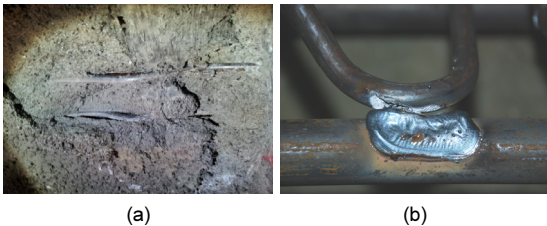
Fig. 3. Weak point of lattice girder : (a) Collapses of lattice girder, (b) Broken welding (Korea Expressway Corporation, 2009)
