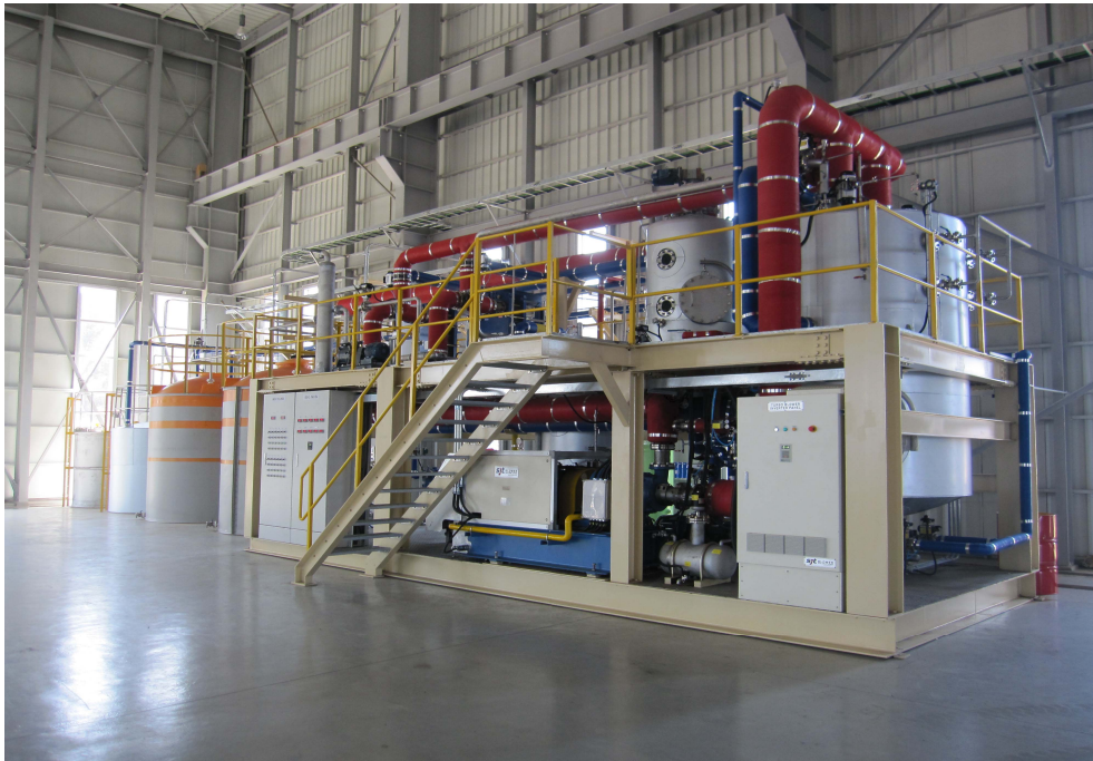
Fig. 3. MVR Desalination Plant
