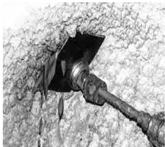
Fig. 1. Leakage of grouting filler
