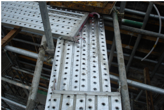
[Figure 5] Faulty of walk plate installation
