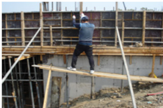
[Figure 6] Faulty of walk plate materials
