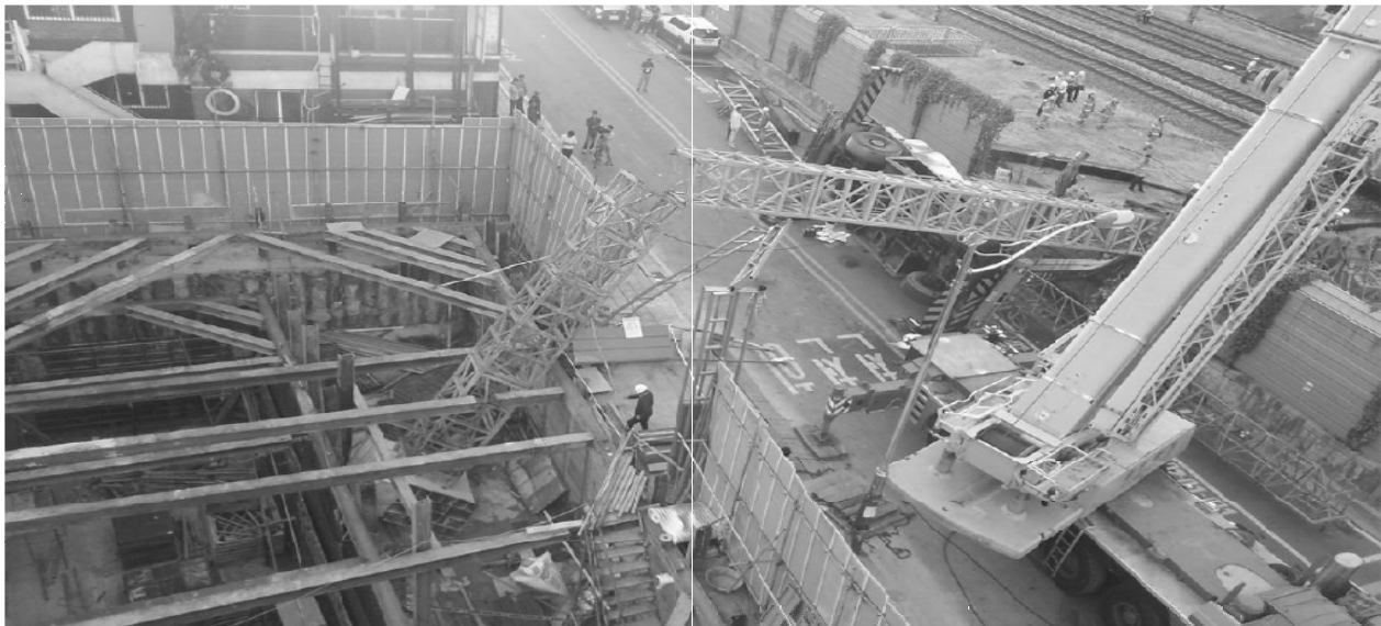
[Figure 1] Incident of Tower Crane at Bupyeong Substation
