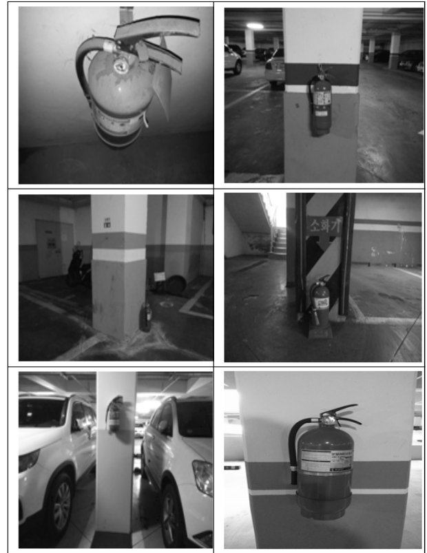
[Figure 1] The installed fire extinguishers
