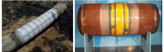
Fig. 9. Installation of composite sleeve(left) and hydraulic test result after composite sleeve repair.
