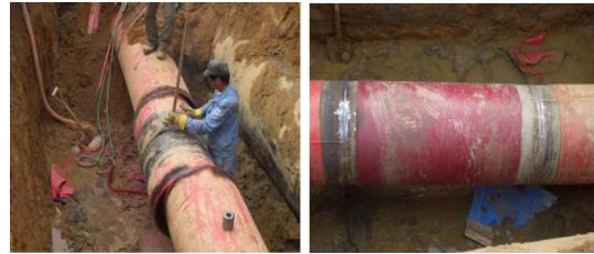
Fig. 4. An example of cutting the defected pipe and replacing with new pipe.
