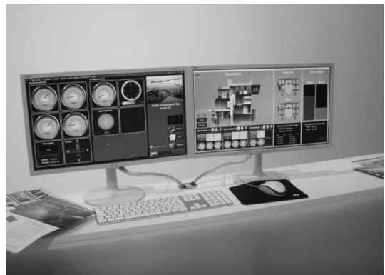
[Fig. 8] Operating and monitoring system for Feed barge
