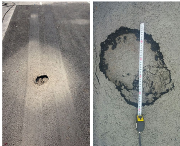
Fig 11. Pavement Collapse in Cavity A
