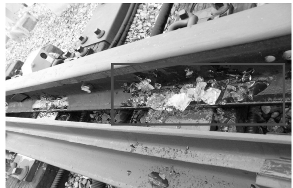
Fig. 6. Stress condition(ice obstruction)
