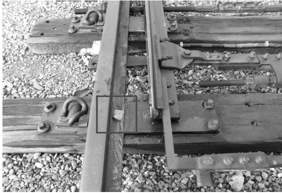
Fig. 7. Stress condition(gravel obstruction)
