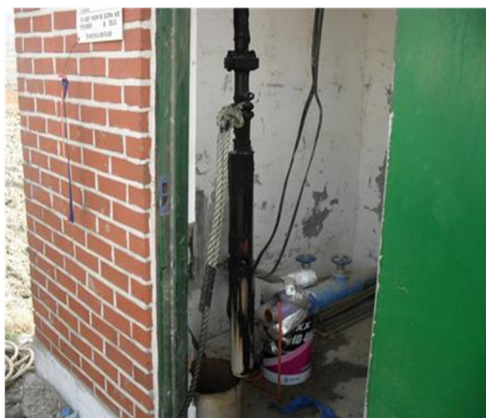
(c) Chemical precipitations on the pumping facilities
