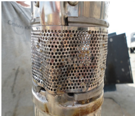
(b) Sand colgging at surface of submerged groundwater pump
