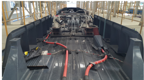
Fig. 3. Detachment of pantograph cover (front view).
