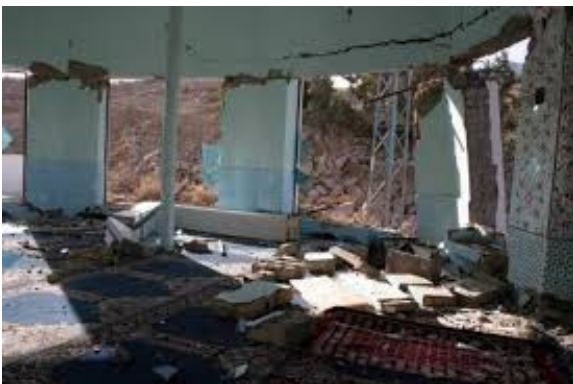
Fig. 2. Seismic failure of masonry pier
