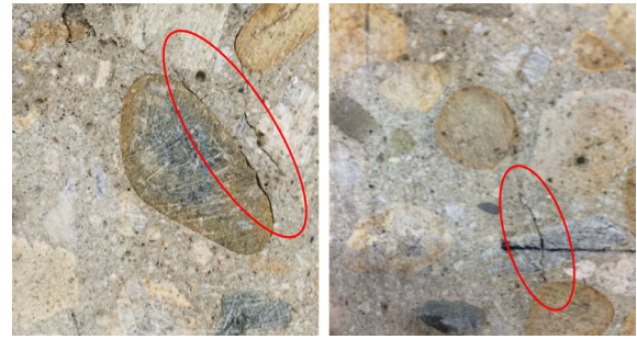
Fig. 10 Cracks around aggregates
