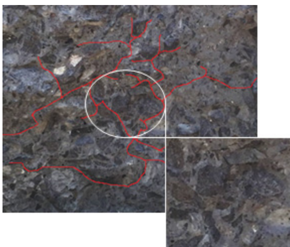
Fig. 5 Typical crack propagation at the failure surface of HWC with f_{ck} of 58.4 MPa
