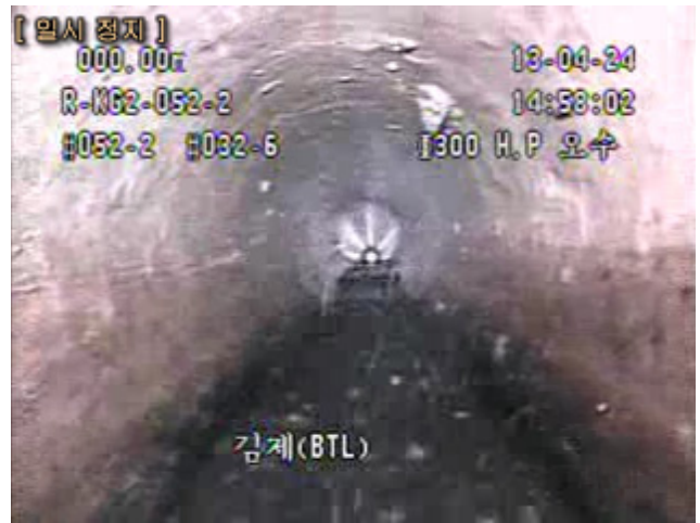
Fig. 1 Sewer CCTV Image
