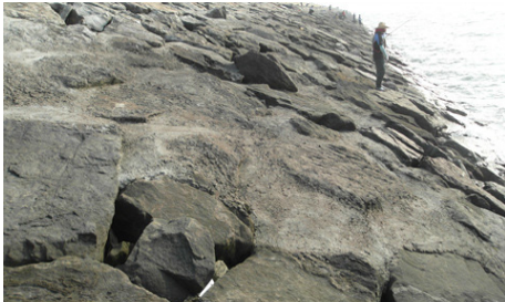
Fig. 9 State of armor stone reinforcement (Siwha)
