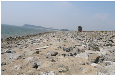
Fig. 10 State of armor stone reinforcement (Nampo)
