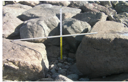
Fig. 7 Deviation of armor stones (Seadike 1)
