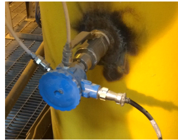
Fig. 10. Measurement system installed in the straight pipe of pulverized coal
