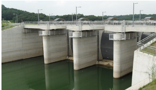
(e) Spillway and slope failure
