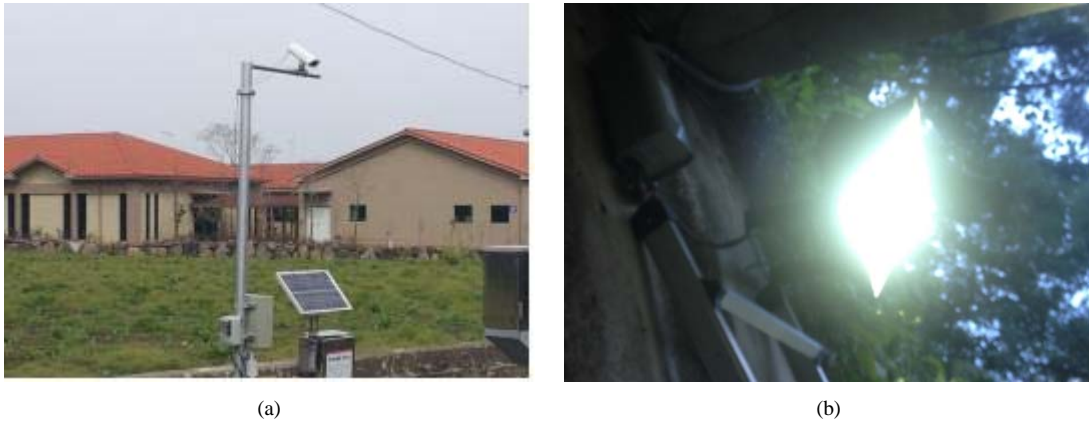
Fig. 3. CCTV system for outflow of the image acquisition at Seong-eup bridge; (a) CCTV; (b) the illumination equipment.
