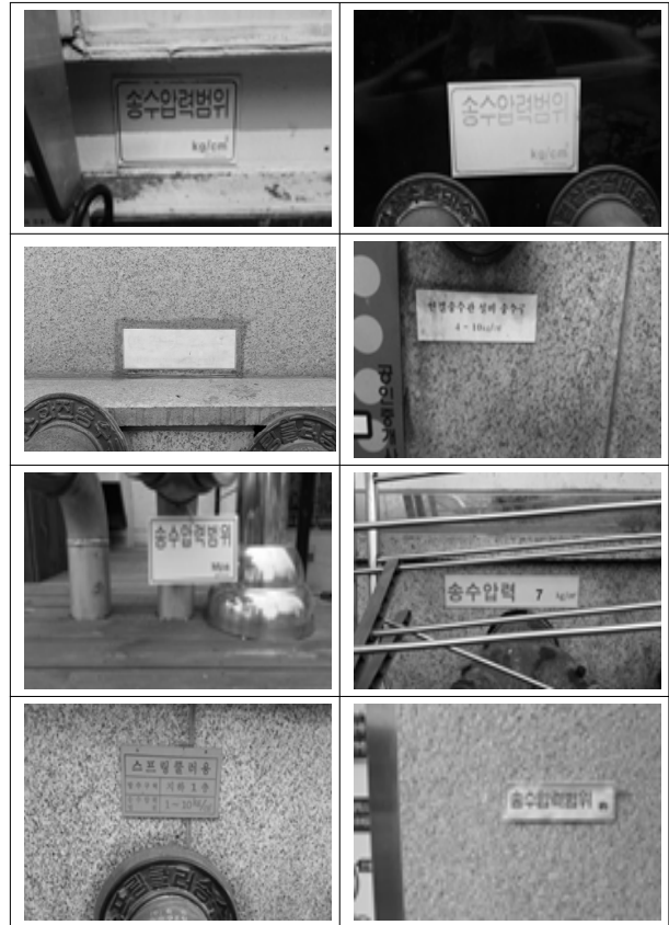
[Figure 8] The attached pressure signs of the fire department connection
