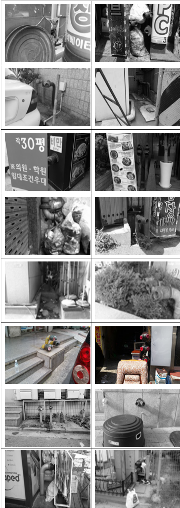
[Figure 7] The fire department connections at the shopping center building
