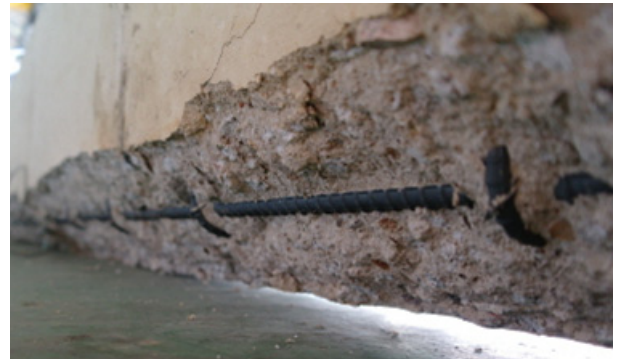
Fig. 20 Exposed steel bars after fire exposure
